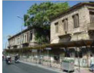
Neoclassical buildings in the center in decay
